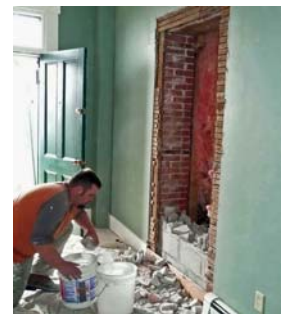
The doorway between the Keeper house and the Electrical room is being “uncovered” by one of David LaMontain’s employees.
