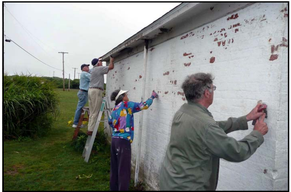
Oil House restoration is well underway thanks to BLMA volunteers headed up by Guy Archambault. Keith Lescarbeau, President of Abcore Restoration has provided guidance. Pictured above are Don O'Laughlin, Charlie Osenton, Wenxian and Richard Calabro.
